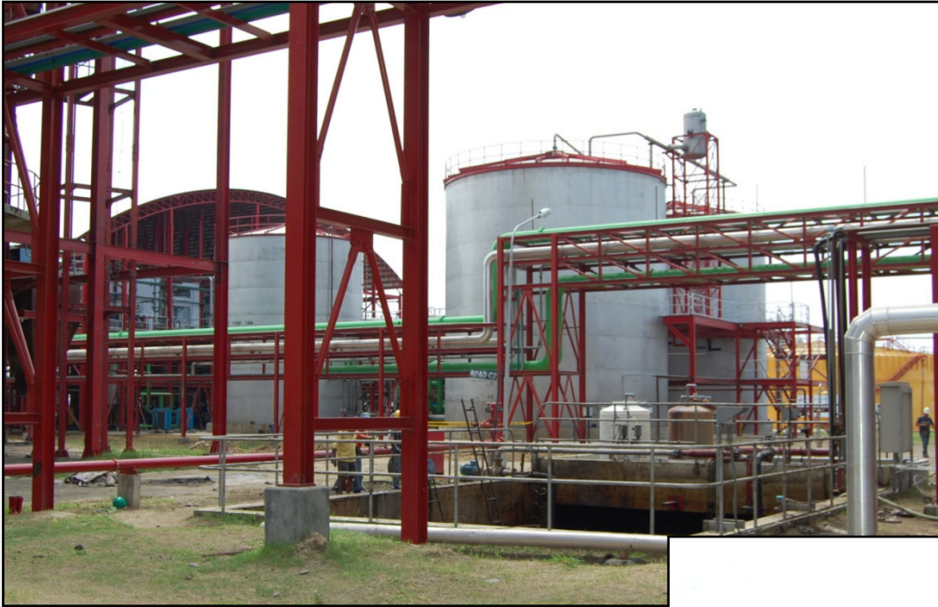
➤ Fuel Ethanol Distillery Plant (SCBI)
